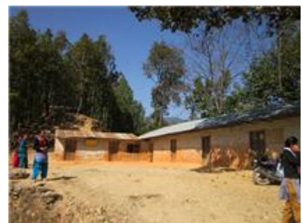
One of the existing school buildings in poor condition.
